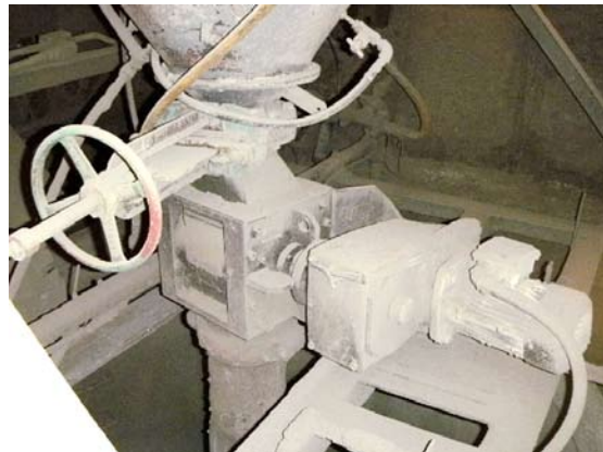
Figure 1. Cement Plant Rotary Valve at the Galena Mine in Idaho (Tight Fit with not a lot of extra working room)
